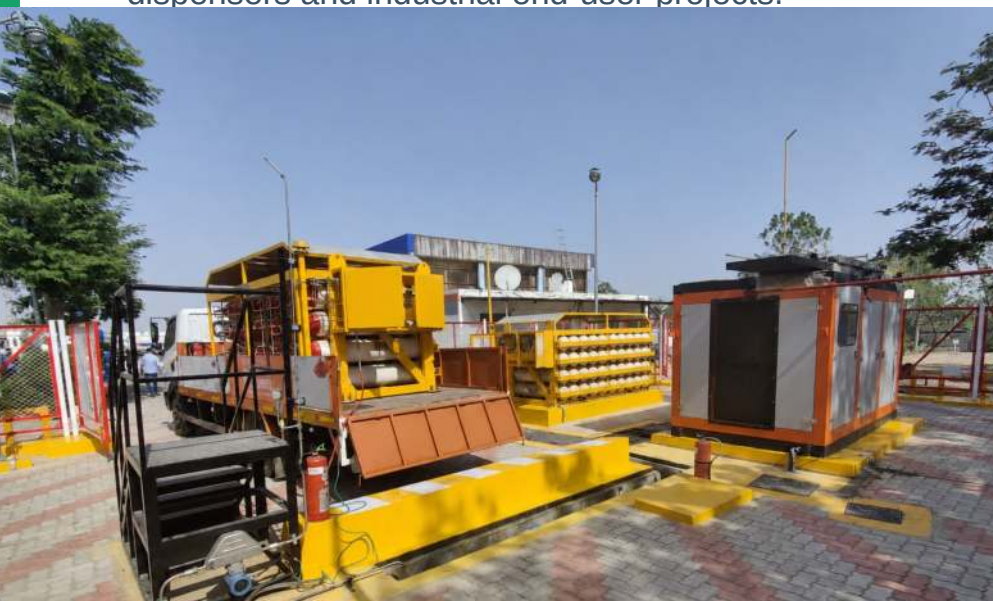
BOOSTER COMPRESSOR • CASCADE • NGV
