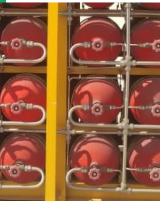
CNG STORAGE & DISTRIBUTION
